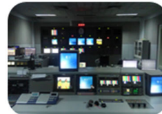
Broadcasting & ICT •Digital Terrestrial Broadcasting •Disaster Information System
