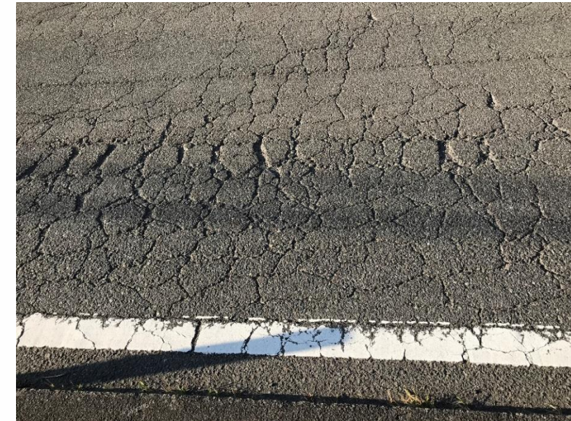
Damaged Paved Road
