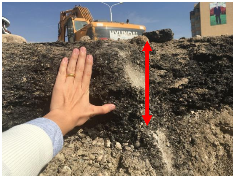
Quite thick asphalt pavement Because of overlay
