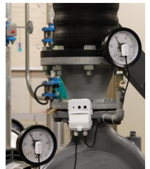
Monitoring analog meter by using magnetic sensor
